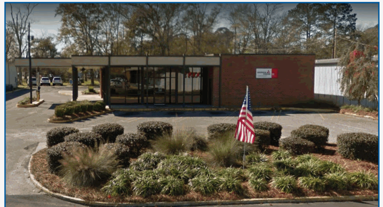
Renovations are underway to convert the old Georgia Power building in Jesup into the newest Marshland Community branch
